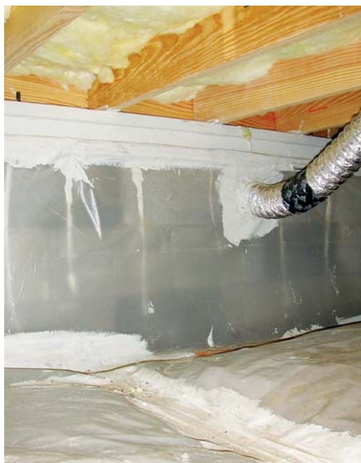
This floor-insulated crawlspace has a termite inspection gap at the top of the vapor retarder. Note that penetrations are thoroughly sealed with mastic.
