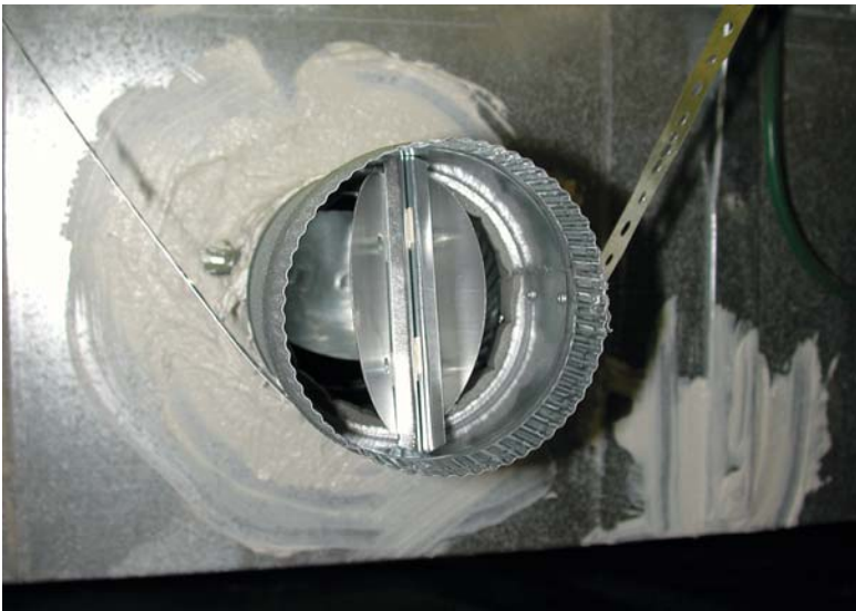
The butterfly damper of this crawlspace supply opens while the system is running. The assembly is sealed with mastic and supported by strapping to ensure that the butterfly damper continues to operate properly.
